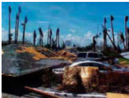
Roofs on the parking garages at the Venetian Terrace Condominium Association in Boynton Beach, Florida, were lifted and collapsed by Hurricane Wilma's winds.
